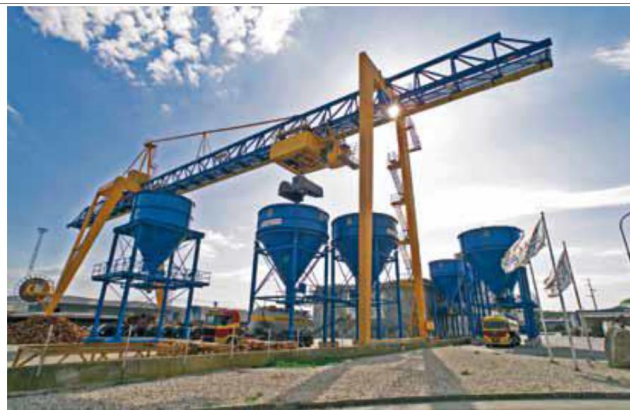
Figure 9: Loading hopper at the port of Krems (source: Mierka Donauhafen Krems)
